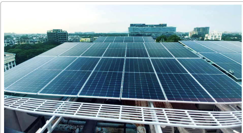
Solar power plant at our Head Office, Pune
