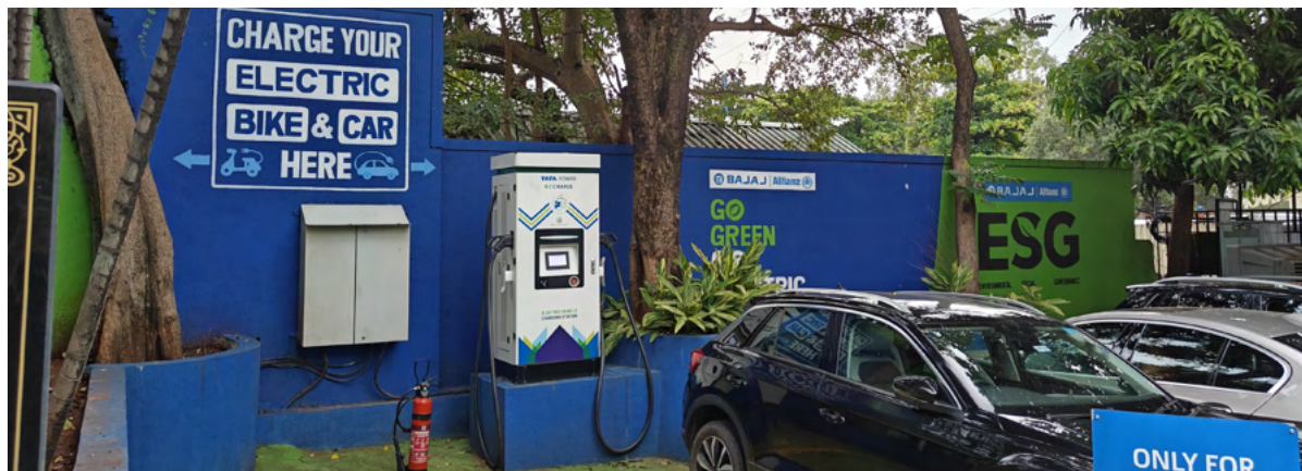
Electric Vehicle Charging facility at our Head Office, Pune
